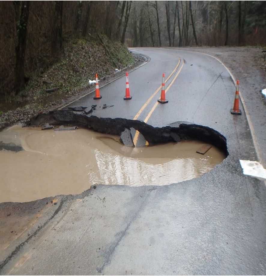
Extreme Rain, Snow and Flooding
